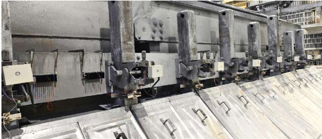
Installation of 16 Wi-Fi enabled data acquisition system and TEG Module
